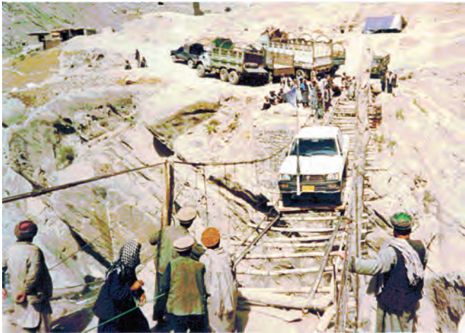
Passage between Fayzabad en Talogan in the North of Afghanistan. Trucks are unloaded at one side of the temporary bridge. Goods are placed on pallets and pulled to the other side. Maximum capacity is 1.000 kg but exceptions are made for 4WD vehicles, preferably without drivers behind the wheel!
